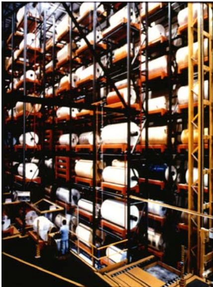
Figure 13.56. Unit Load Automated Storage/Retrieval System for Paper Rolls
