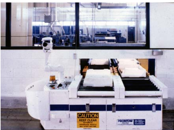
Figure 13.41. Multiload AGVS Interfacing with a Clean Room
